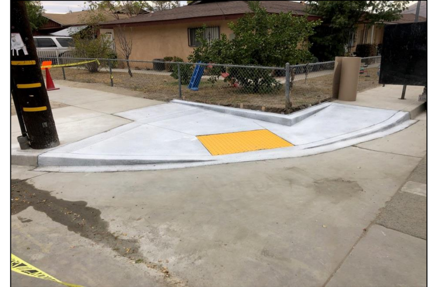
A new ADA ramp and sidewalk was installed at 1 st and Jordan
