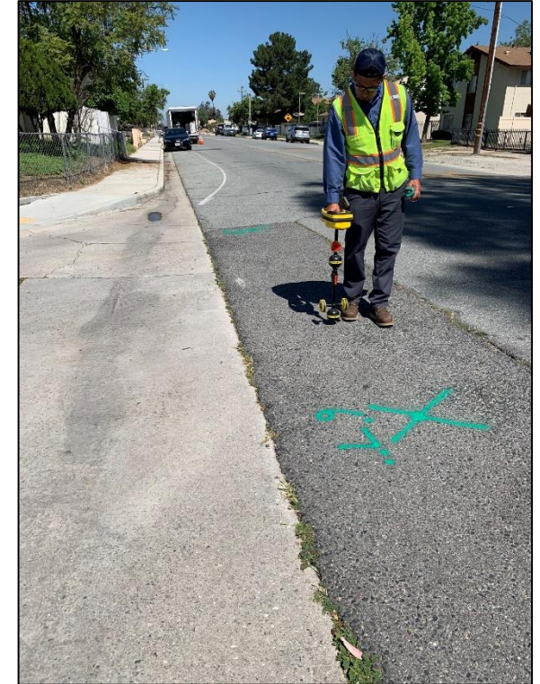
Located and marked sewer lines in response to a Dig Alert request
