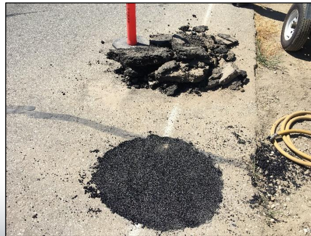
Exposed & re-compacted sink hole on Sanderson Ave
