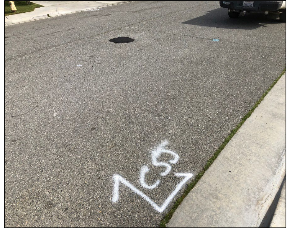
Crew responded to sinkhole at 2774 Burgundy Lace Lane
