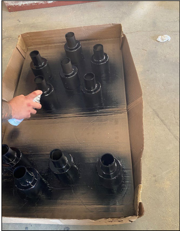
Preparing solar lights for installation at Rancho San Jacinto Basins and Channels
